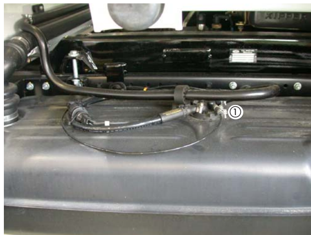
① Steigrohr, eingebaut in der Tankarmatur Rising pipe, installed in the tank fitting
